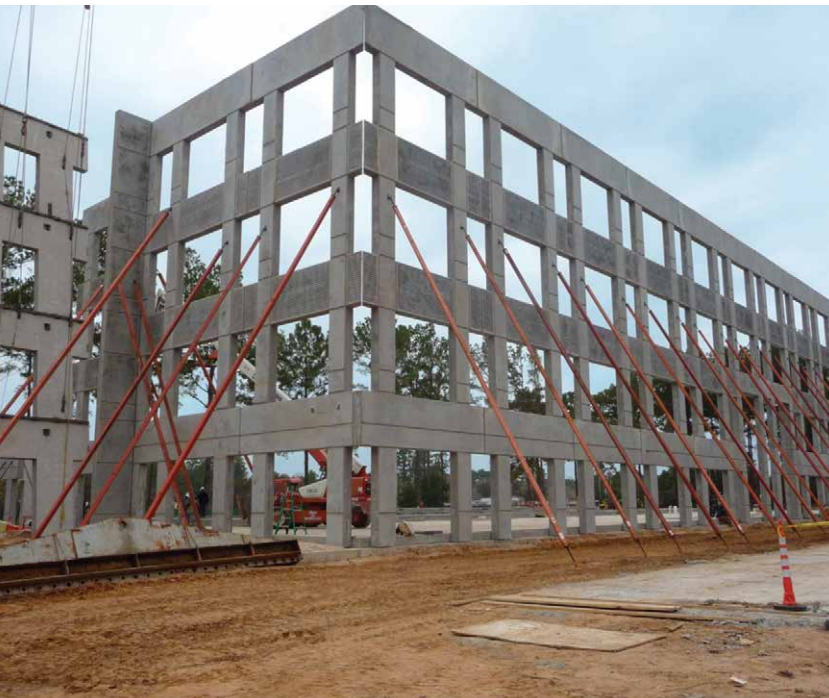
Using 42' Accubrace instead of the originally planned 52' other braces meant more room around the tight site for the crane to move, and lower shipping costs.
