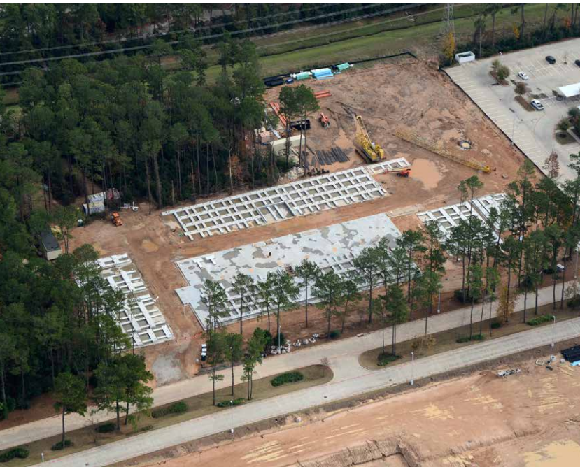
The original plans were scrapped and new panel layouts were created in just days in order to allow the contractor to switch to Accubrace braces and reap savings in time, equipment rental, and shipping costs. (Photo courtesy of Aero Photos)
