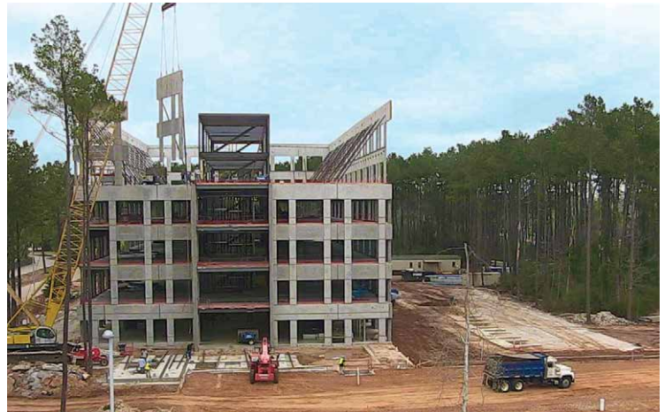
Stacking tilt-up panels is becoming a more common practice as more architects design taller tilt-up structures.
