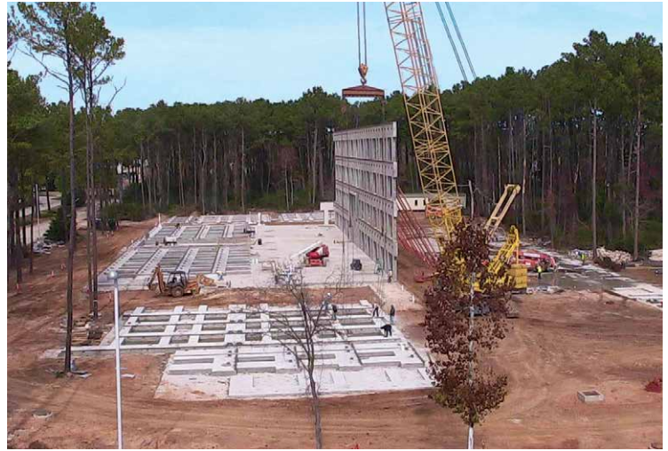
The panel book includes panel designs, insert locations, and other details that helped this project move quickly from the first day.
