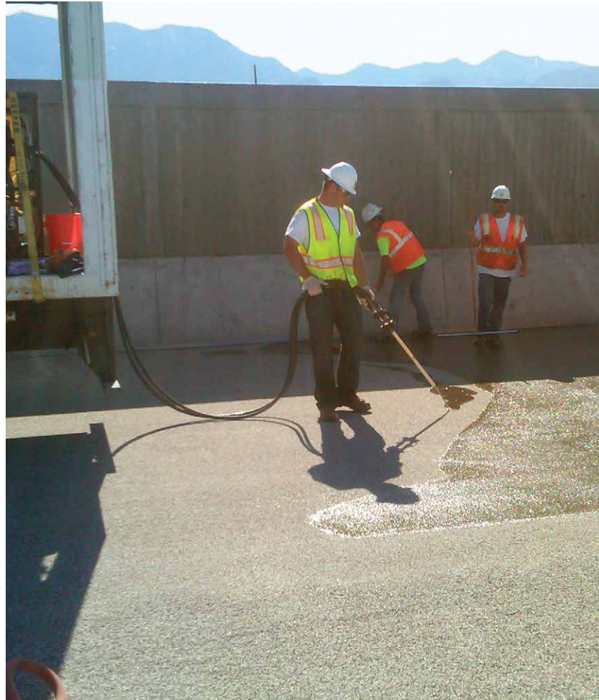
Unitex devised a pump system for this project, training the operator to provide the optimal application.
