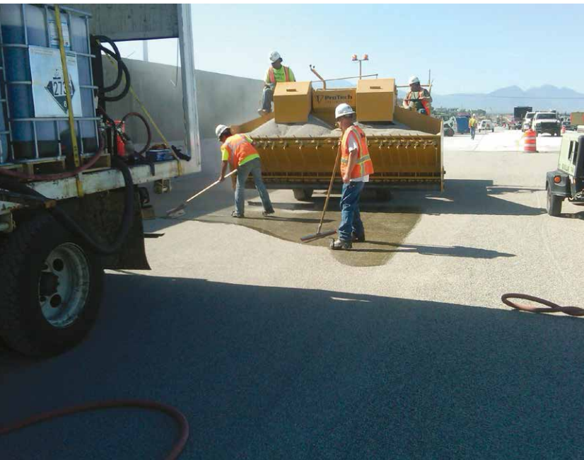
ProTech and Unitex worked together to create a product to meet the demanding UDOT criteria for protecting the surface of 55 new bridges to help them withstand extreme weather and heavy traffic conditions.
