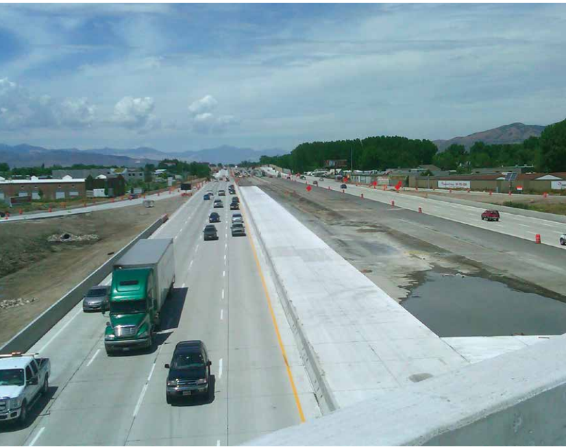
Expanding and improving the I-15 Corridor to encourage economic growth and handle projected traffic economically meant that concrete pavement was widened and the road surface of replaced bridges would be treated to withstand demanding conditions.
