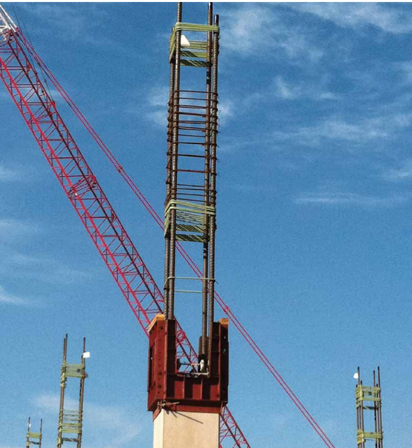
With a large number of tapered rebar ends to create, Ambassador Steel appreciated the speed and quality they achieved with the Taper-Lock Machine.
