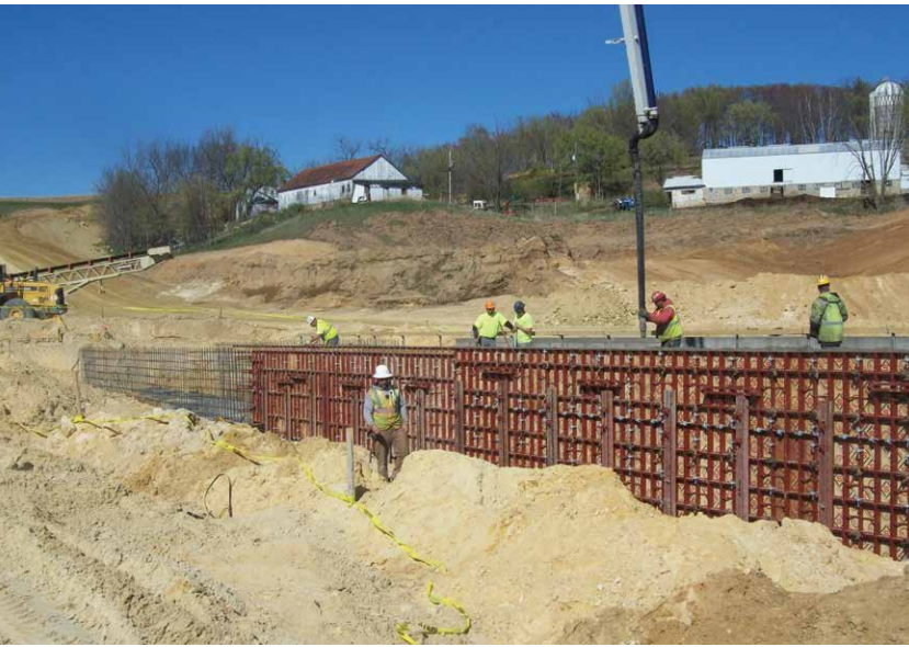
Cycling gangs of forms through a number of pours allows contractors to reduce materials needed on the job site.
