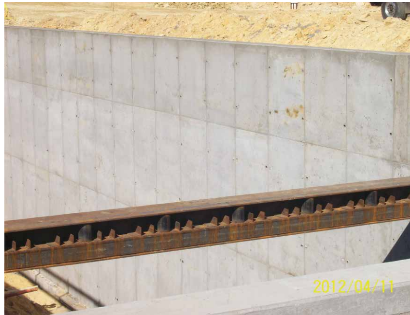
The Sym-Ply gangs required just two Taper Ties per form, speeding construction and reducing the material list.
