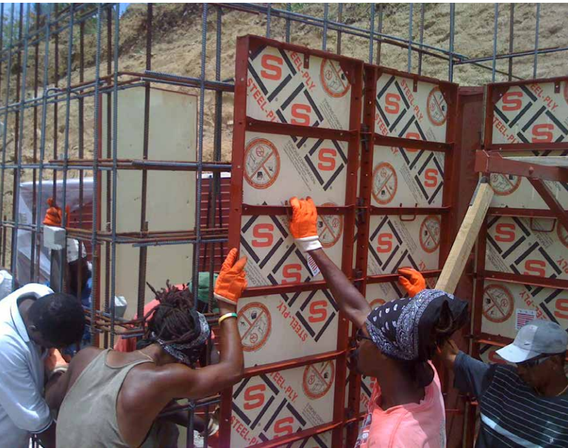
No crane was required for setting the forms. Workers were able to hand set forms very simply.
