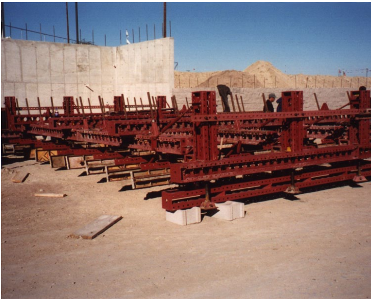
The 20' wide system was designed to roll from one location to another for multiple reuses.
