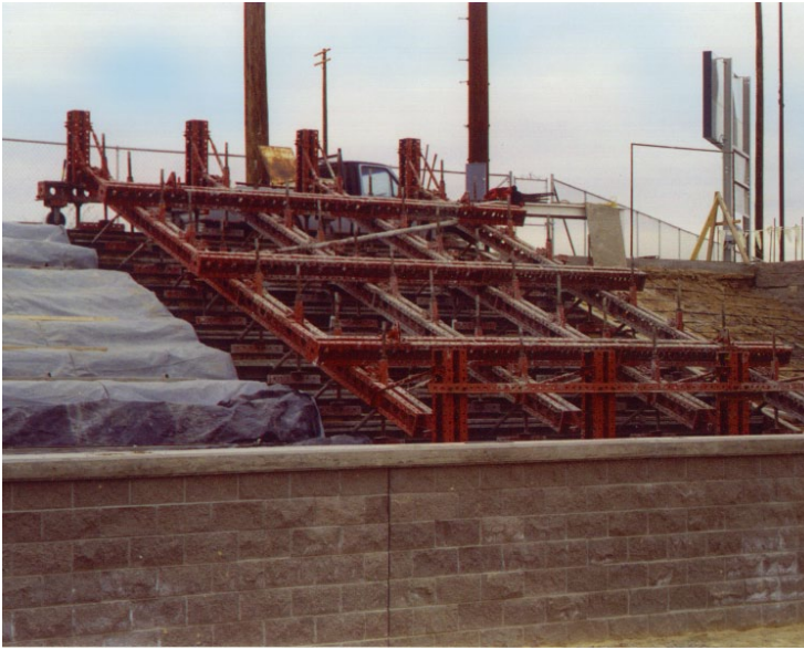
A grid of Symons Soldiers and Max-A-Form components supported the Steel-Ply forms for the high school stadium project.
