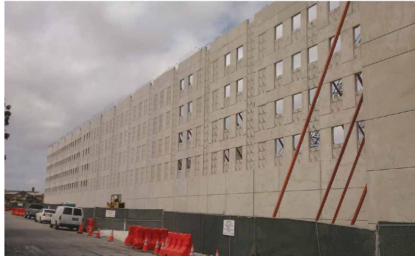
The contractor did not want to have to find room for a large crane on this tight job site or pay the high rent for one, so a plan was devised to reduce the panel height and join the stacked panels with Sleeve-Lock.
