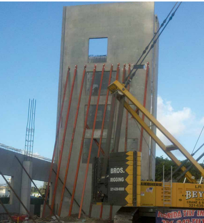
Just 10 Accubrace supports were required for this very tall panel to meet hurricane wind load requirements.
