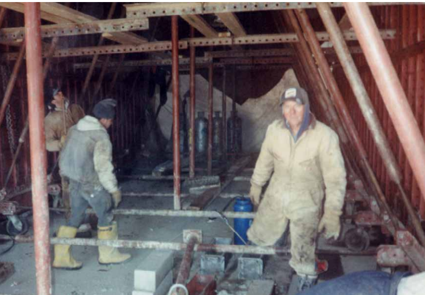
An unusually large overall size, very thick walls and overhead slab, site conditions and cold weather combined to make constructing a simple access tunnel into a forming challenge.
