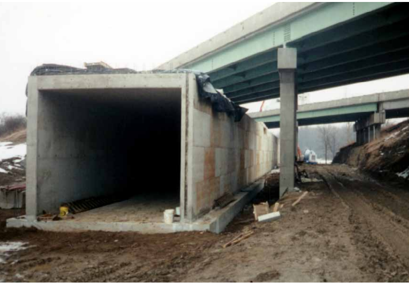
Exceptionally wide access tunnel design required an additional center slab support provided by Post Shores.
