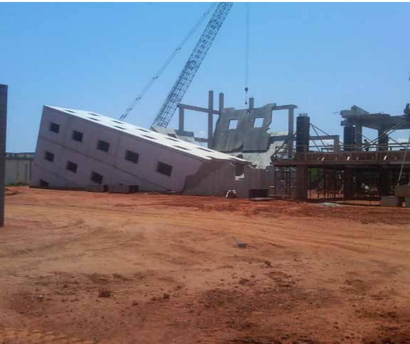
Tilt-up construction is typically designed for structures that are constructed in plumb, so this project presented unique challenges.
