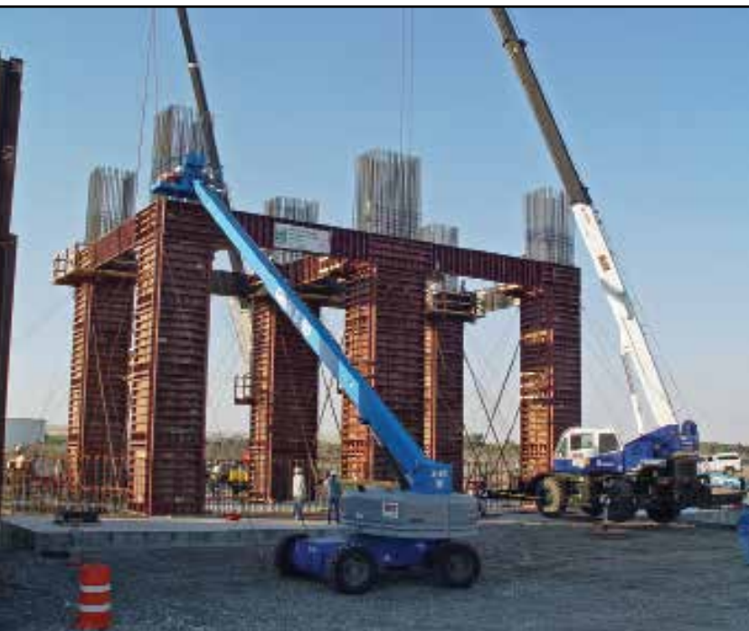
The second stage of the coker construction was the construction of the 36' tall, 6' x 6' and 6' x 8', columns.
