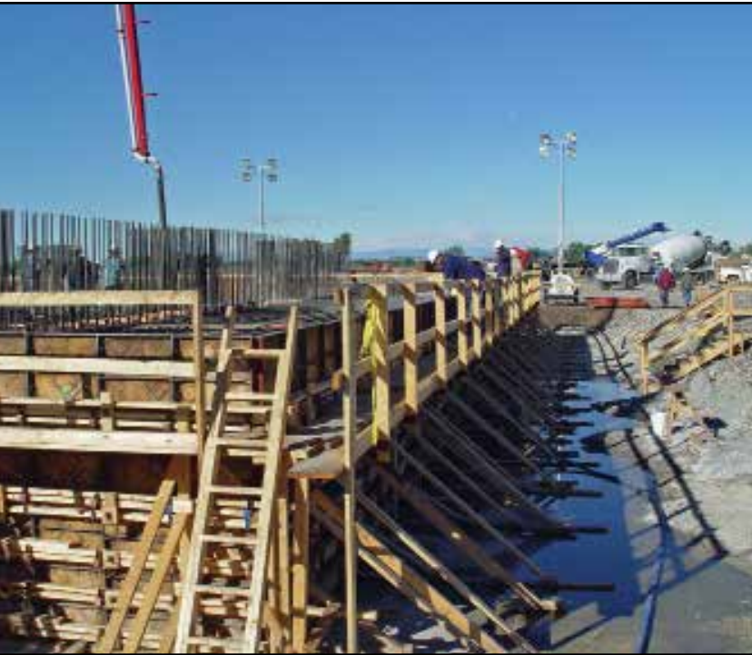
The 60' x 90' x 7' thick concrete pad was designed to support the massive structure and coker equipment.
