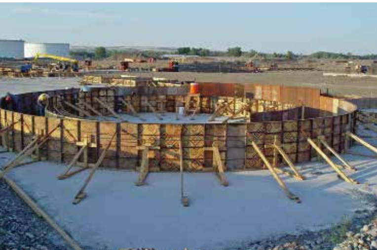
Panels 4' high formed the circular footing for a new storage tank at the facility.
