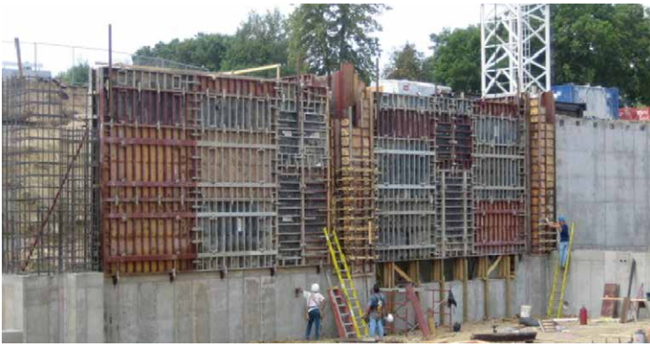
The Rapid Clamp system was used in the straight sections of the wall and the Steel-Ply system on the pilasters and smaller areas.
