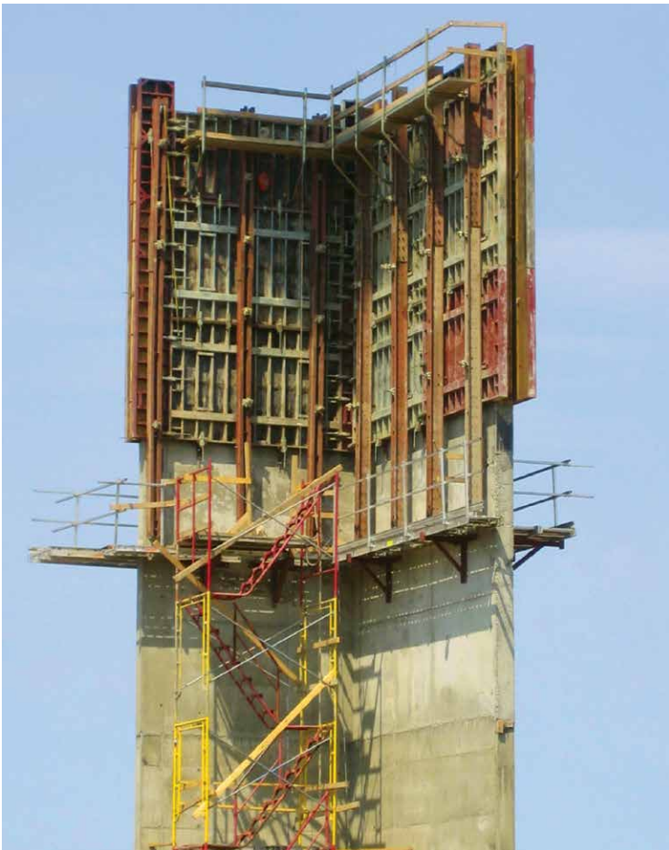
The shearwalls were formed using with gangs of forms on Support Brackets (since discontinued) with trailing steel walers for alignment.
