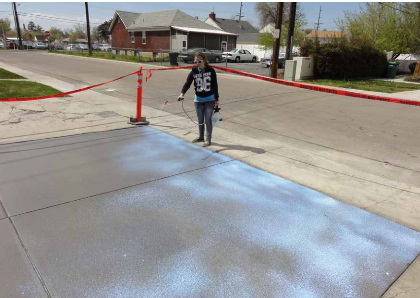
Students from the BYU Civil and Environmental Engineering program participated in a service learning project to replace a concrete driveway.
