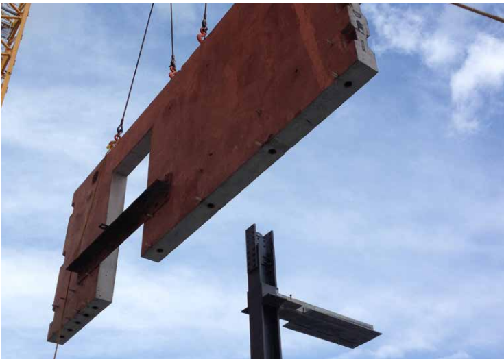
Concrete walls were precast with a Sleeve-Lock rebar coupler along the bottom edge, ready to connect Dowel Bars and Dowel-Ins..
