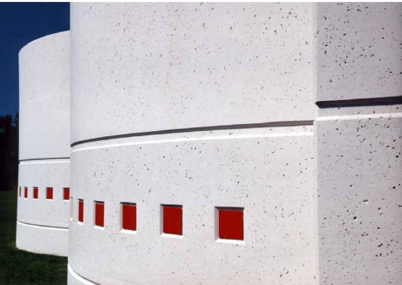
The wall was enhanced with surface detail provided by rustication strips, an acrylic coating and colorful reglets.
