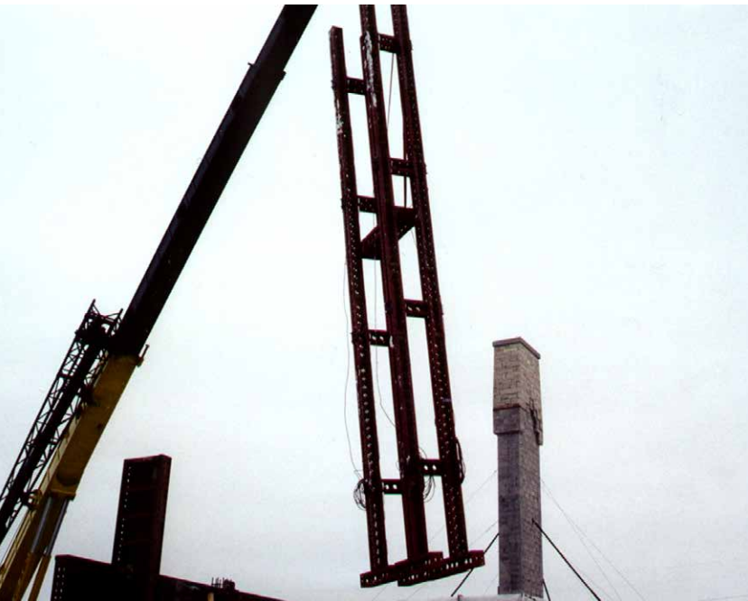
The center shoring tower provided alignment for the column forms and support for the cap form.
