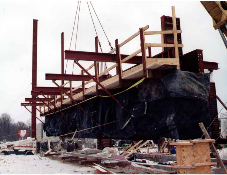
The 64' long cap assembly included a working platform and a hinged soffit.
