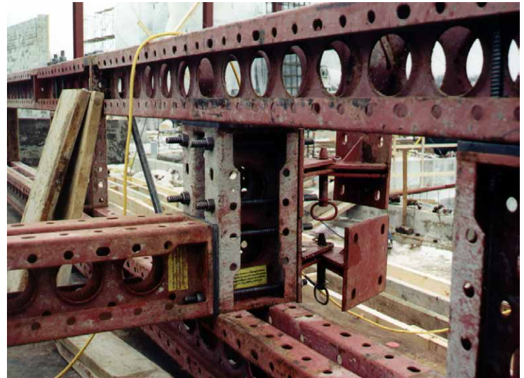
Assembling form and shoring components in sections on the ground minimized expensive crane time.
