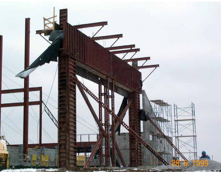
The completely assembled forming system allowed the contractor to pour the entire proscenium without ties. The detailed form assembly plans from Symons ensured a precise fit between all components.
