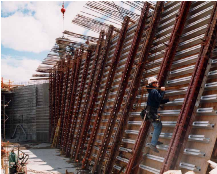
Symons Soldier was used as walers to carry the Taper Tie loads for the Aluminum Beam Gang system.
