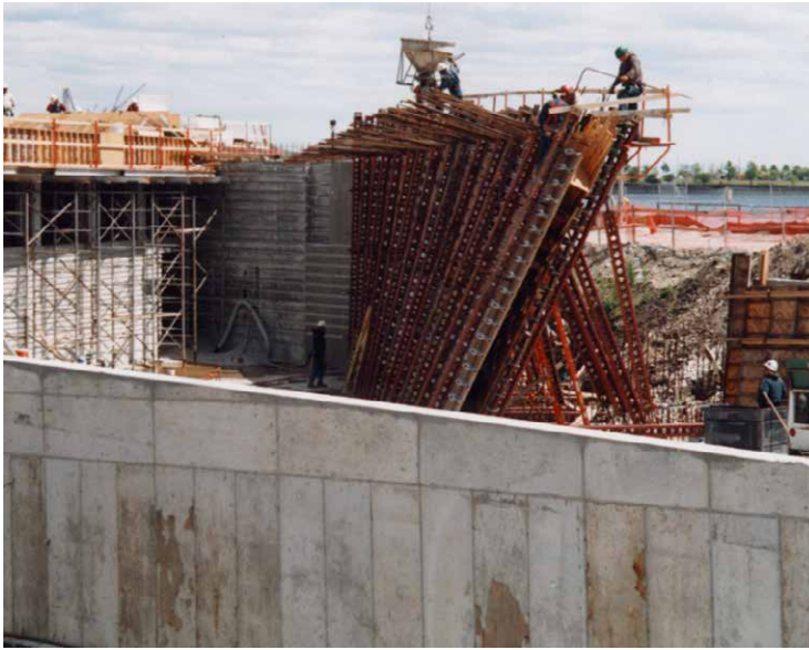
The concrete retaining wall was designed with a 25° twist that posed some unusual forming challenges.
