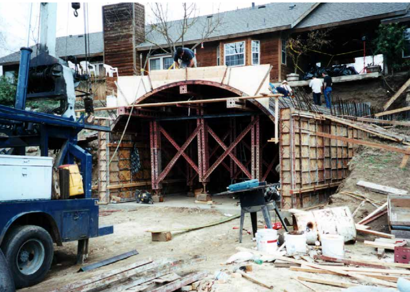
Symons provided detailed plans that combined several forming systems and shoring to form the structure monolithically.
