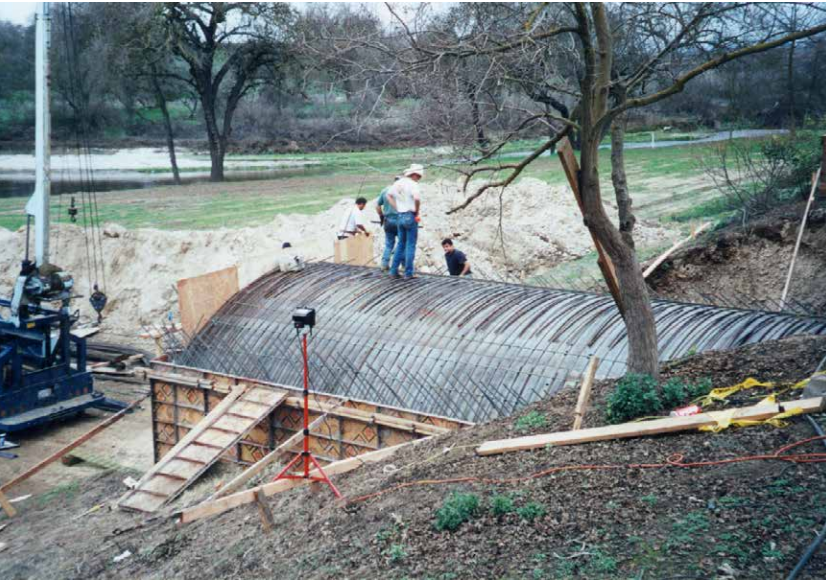
The architect designed the hillside storage building with an arched roof to withstand the weight of the soil.
