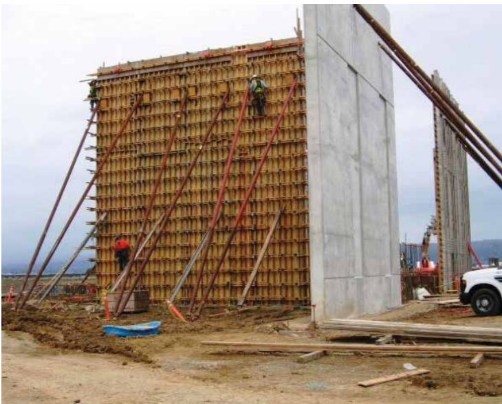
A panel prior to removing the forms alongside two panels with forms removed.
