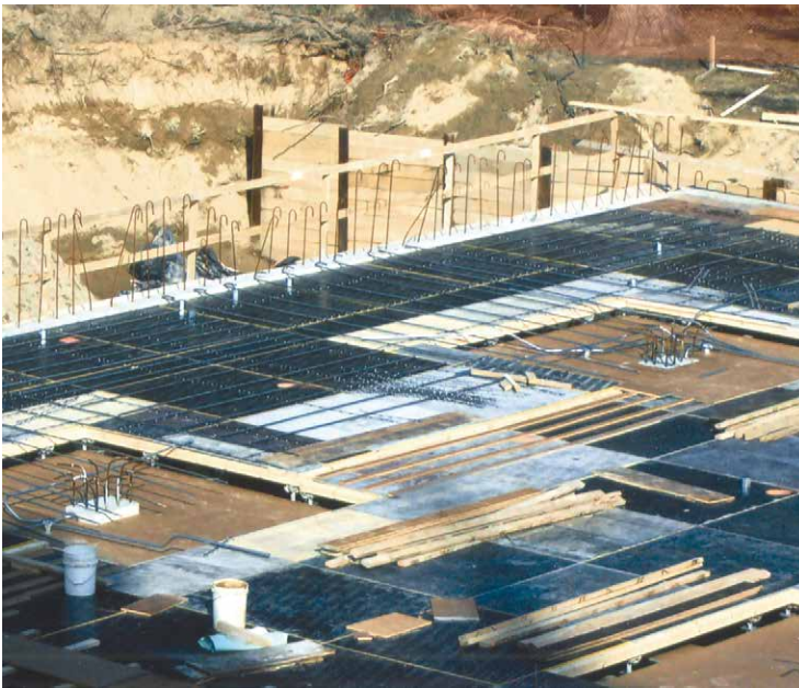
Utilizing a combination of large panels and fillers, the contractor could accommodate the drop heads and the drainage slopes.
