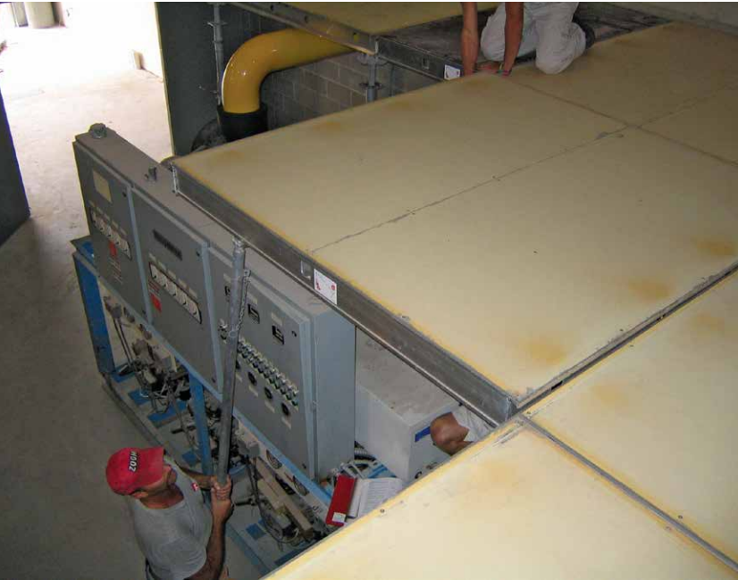
A careful layout allowed the large 180x180 DeckFast panel to span previously installed cooling machinery and pipes.
