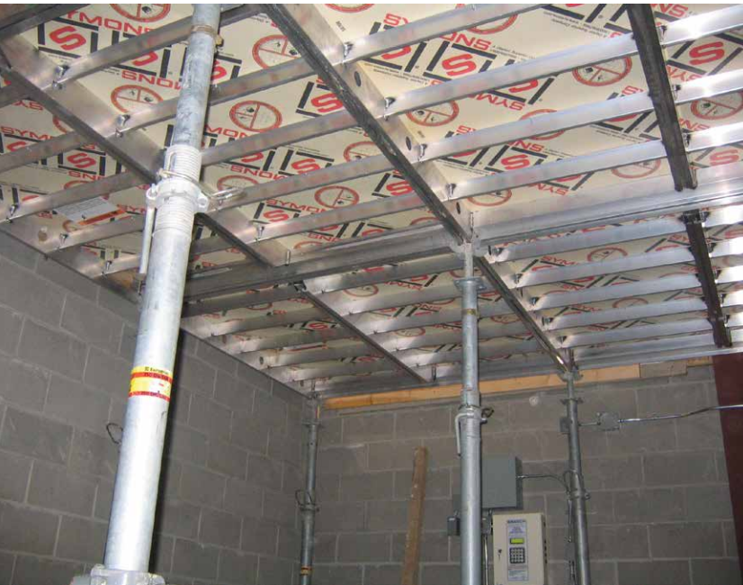
The contractor appreciated the financial benefit of the reusable, rentable DeckFast shoring system.
