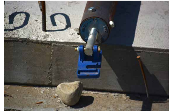
Shoes at the base of each brace attach them to the slab to provide a strong connection.
