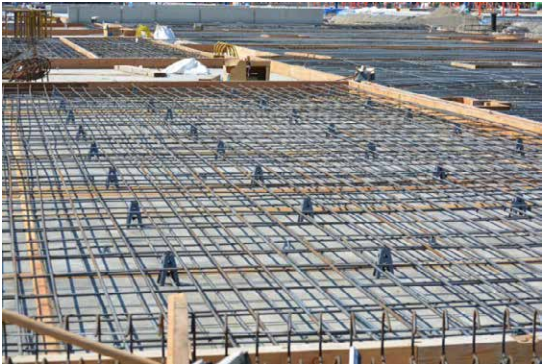
To lift, space and tie rebar, Dayton Superior PEZ E-Z Chair®, the PTZ Tower Chair, PSW Space Wheels and Tie Wire were supplied.
