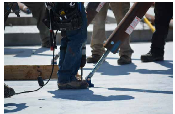
Once the panels are in place, workers fasten braces to the warehouse slab. Braces align and support panels during construction.
