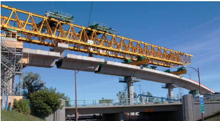
The specialized Segmental Bridge Epoxy was utilized in this rail overpass. (Photo courtesy of CanadaWeb Inc.)
