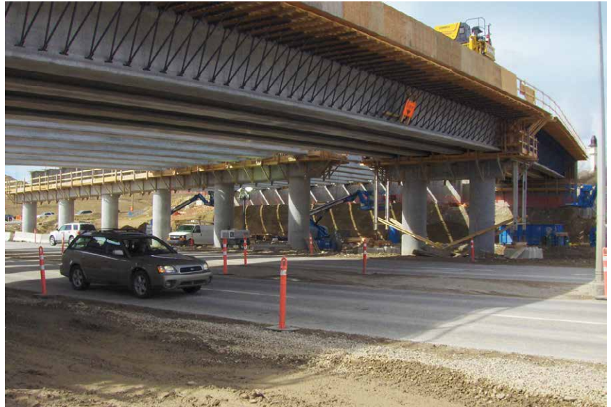
Bridge Overhang Brackets attached to the NU style girders supported the bridge deck during construction. (Photo courtesy of City of Calgary)
