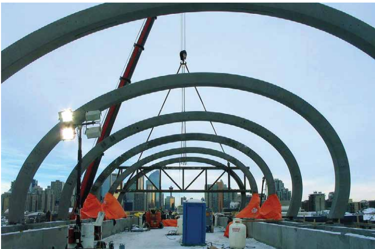
The distinctive roof supports for the new Sunalta train station utilized Bar Lock to join long rebar strands in their rebar cages.
