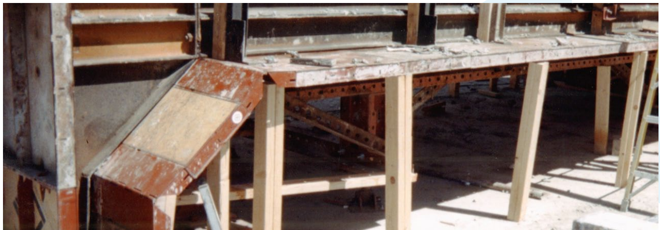
Forms were longer than required for the 7' sections so that workers could have a convenient work area.
