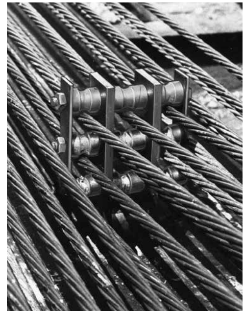
Illustration of swivel action as strand restraining device responds to strand tensioning.
