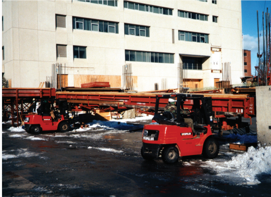
Fork Lifts position steel beam forms between columns, and then workers lower the attached support frames.
