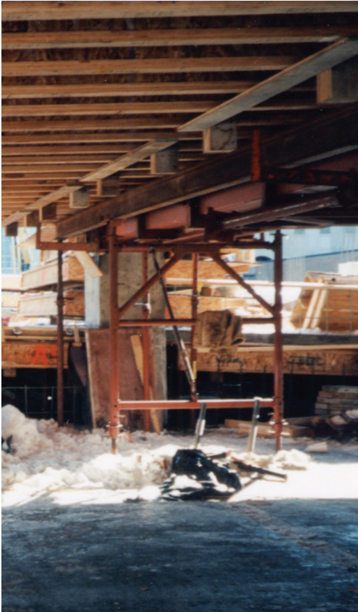
The strong and adjustable load frames with wide deck panels allowed large, clear work spaces for easy accessibility.
