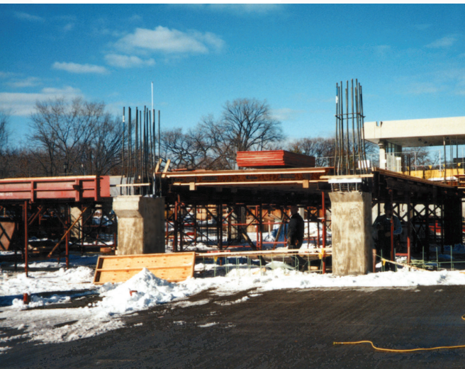
The site was too tight for much crane access, but the Garage Beam System components are placed with forklifts.
