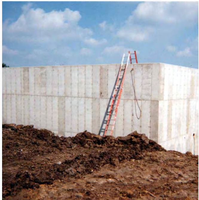
Steel-Ply forms were used in a handset application where muddy conditions did not allow them to place a large crane.
