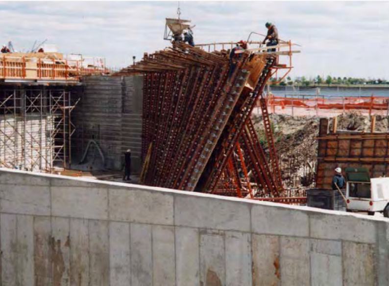
The concrete retaining wall was designed with a 25° twist that posed some unusual forming and support challenges.
