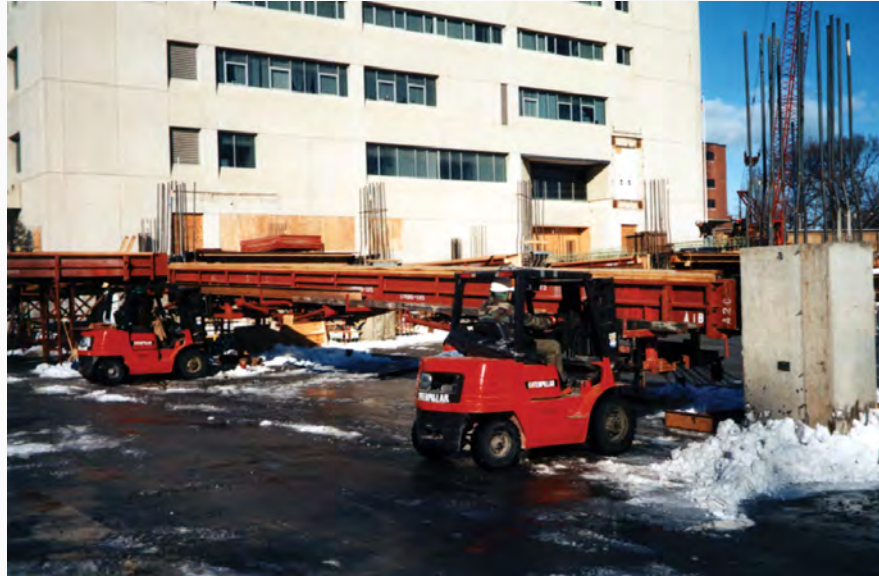
Fork Lifts position steel beam forms between columns, and then workers lower the attached support frames.
