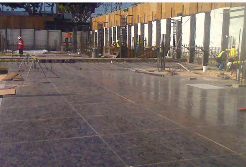
The system was erected at a rate of 160 square feet per manhour despite the crew not being familiar with it initially.
