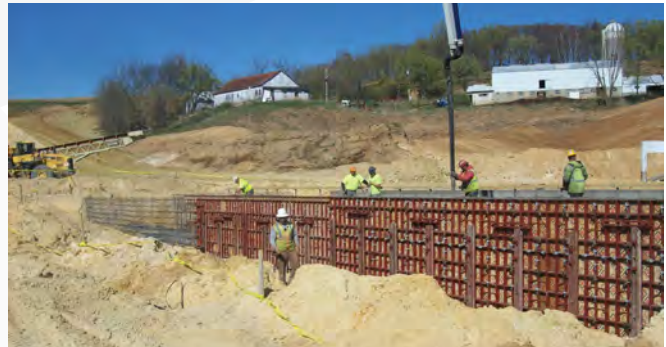
Cycling gangs of forms through a number of pours allows contractors to reduce materials needed on the job site.
