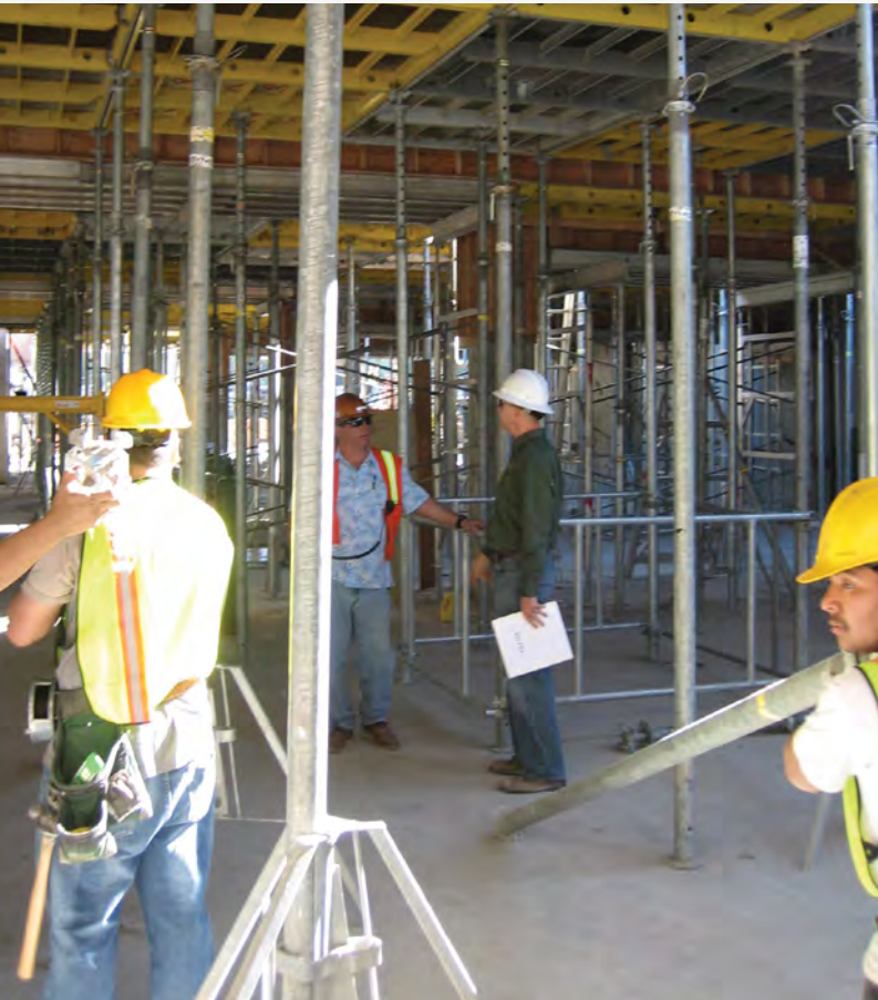
The small crew worked quickly, even at a forming height of twelve feet.
