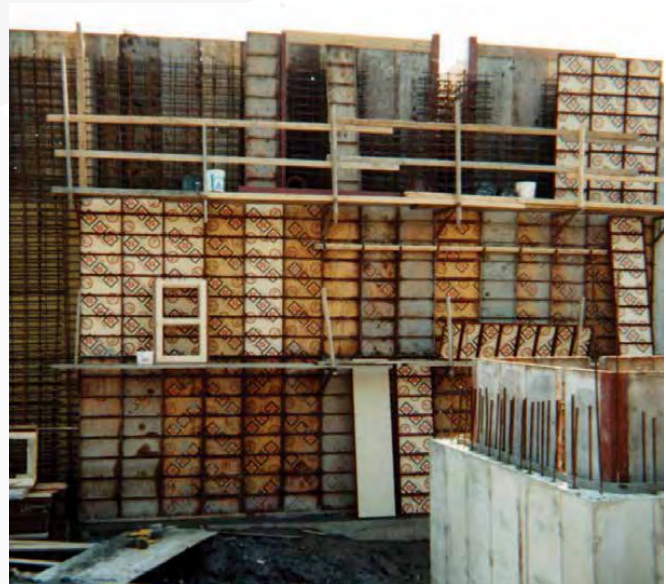
The Steel-Ply forming system was used for foundations and walls throughout this large expansion project.
