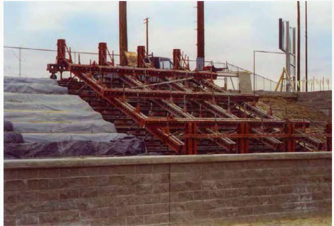
A grid of Symons Soldiers and Max-A-Form components supported the Steel-Ply forms for the high school stadium project.
