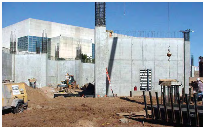
Although the arena design featured columns of many different sizes, the concrete forming systems were easily adapted to each situation.
