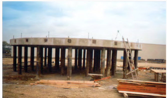
F. W. Johnston Construction felt confident that the success of their first raised platform project helped them expand their business.
