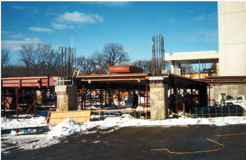
The site was too tight for much crane access, but the Garage Beam System components are placed with forklifts.
