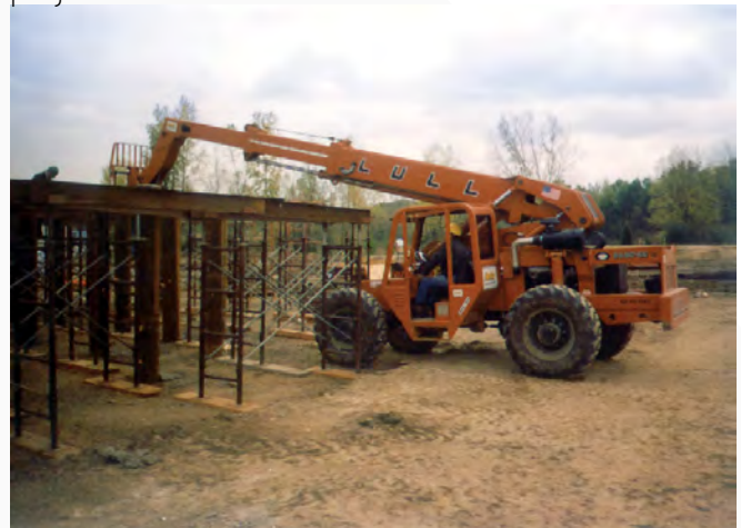
With detailed plans to guide them, the crew was able to quickly set up the shoring system and finish the raised platform ahead of schedule.
