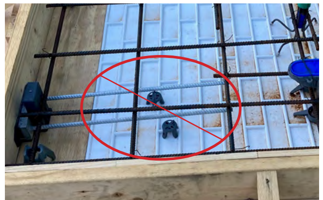
FIGURE 1 - Incorrectly tying in PBA into existing mat
