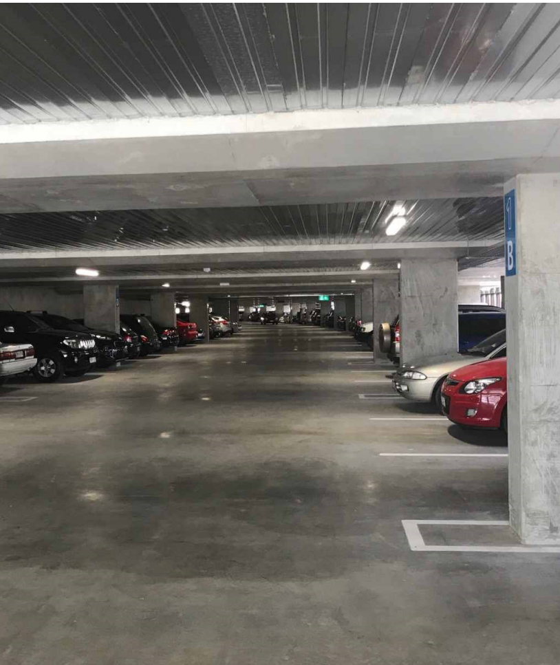
By using Lithium Hardener, the contractor only needed one day per level to treat the concrete, compared to 3-4 day closure required for conventional epoxy or polyurethane coatings.
