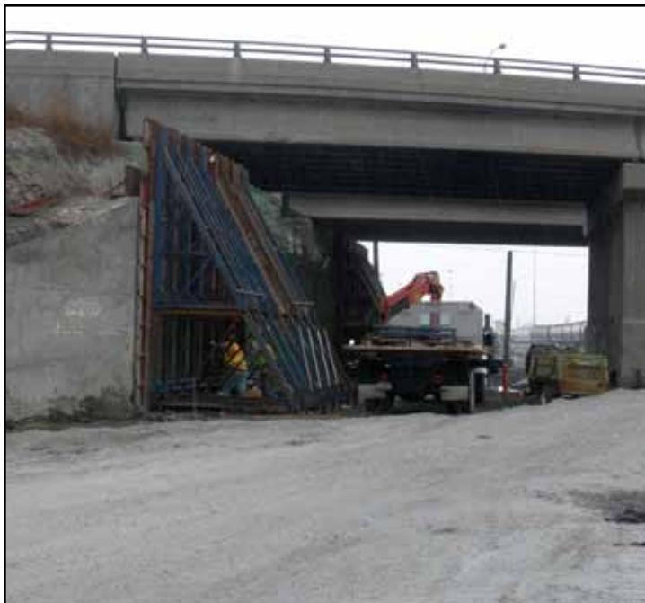
When the new retaining wall was in place, CSX Railway gained the rail yard access that they required.
