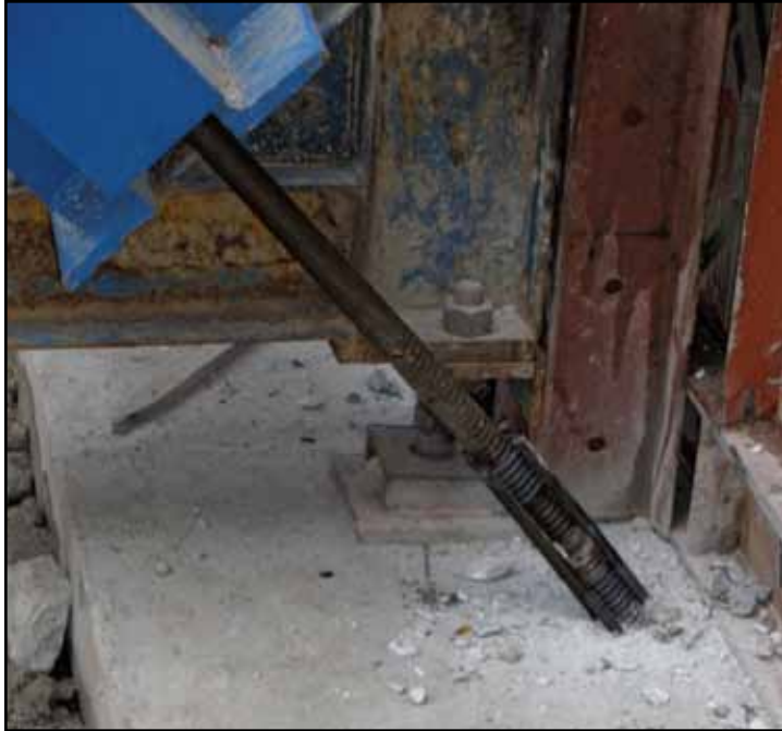
Coil Rod was epoxied into the footings after the frames were in place, so there was never any problem with the Tie Rods.
