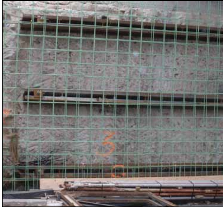
The contractor removed an existing retaining wall to widen access to the rail yard.
