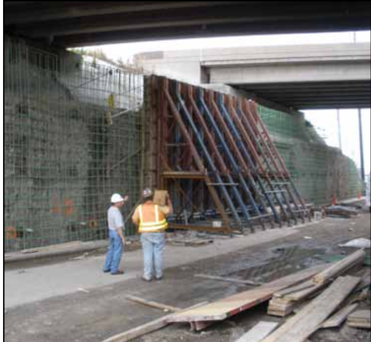
The Backbone frame braced a Steel-Ply gang for this one-sided forming application.
