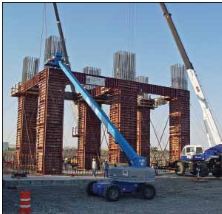
The second stage of the coker construction was the construction of the 36' tall, 6' x 6' and 6' x 8', columns.
