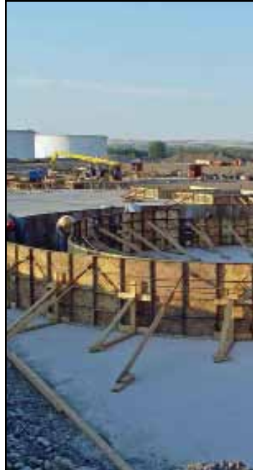
Panels 4' high formed the circular footing for a new storage tank at the facility.
