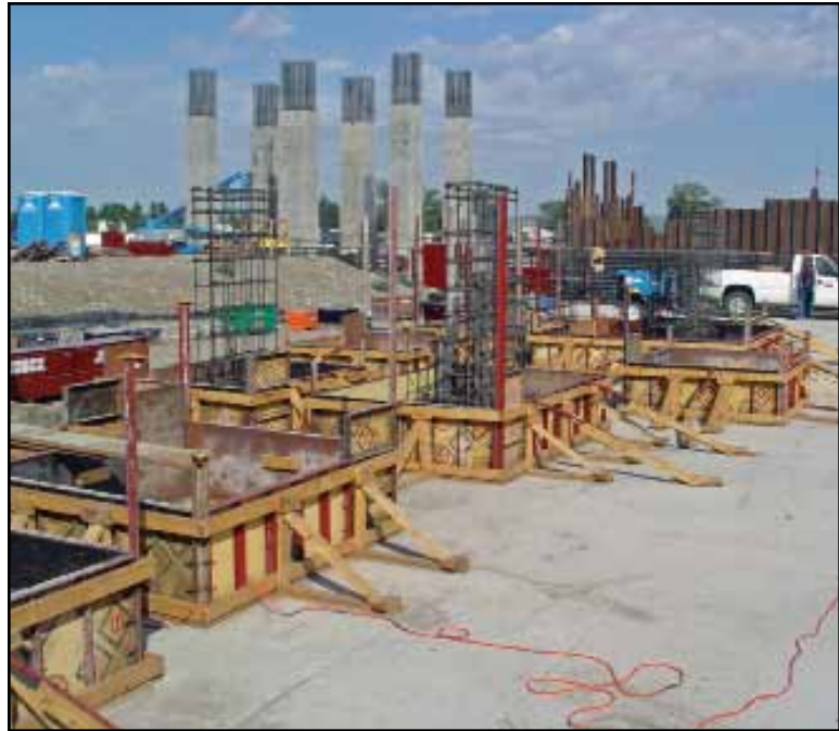
Steel-Ply was used for pads, footings and columns for various structures all over the site.
