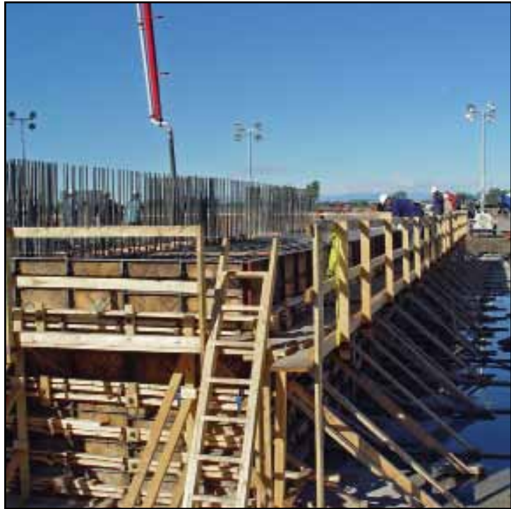
The 60' x 90' x 7' thick concrete pad was designed to support the massive structure and coker equipment.
